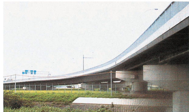
Photo 5 Appearance of World-cup-kyo Bridge applied with Cupten coat M treatment and pre-coat system (Yokohama City)
